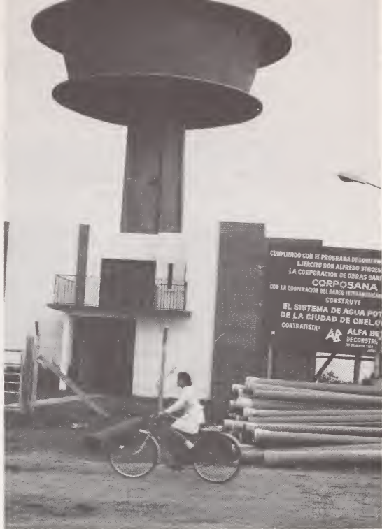
Construction of a water treatment plant at Coronel Oviedo Courtesy Inter-American Development Bank
