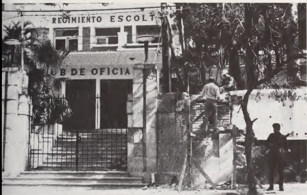
One week after the 1989 coup, workers plaster over bullet holes and repair the front walls of the Presidential Escort Regiment headquarters, Asunción. Courtesy Richard S. Sacks
